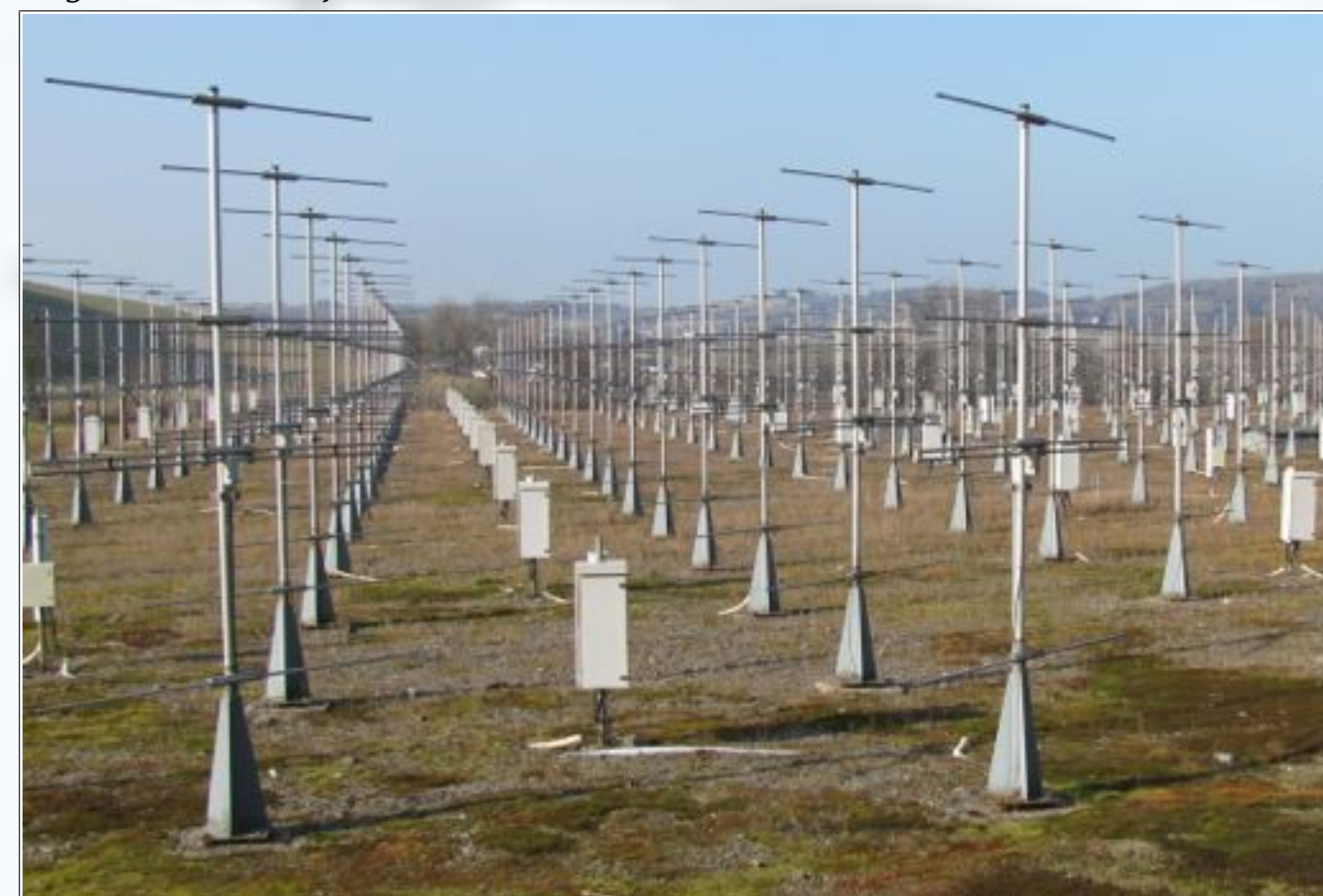
Fig1. Part of the Aberystwyth antenna array showing the original Phase Shifter units
