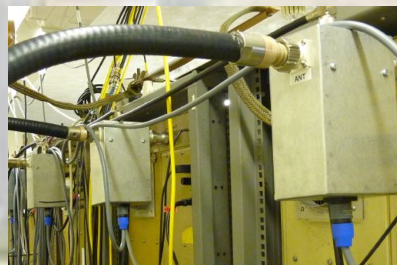
Fig 9. Custom designed multi-couplers installed on the rear of the Aberystwyth Transmitters.
