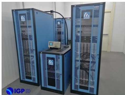
(Above) Another view of the equipment racks for the two 96 kW drivers (Photo credits IGP)
