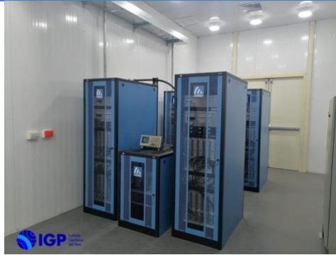
(Above) The equipment racks for the two 96 kW drivers
