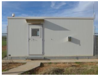
(Above) radar enclosure with interlock fitted
